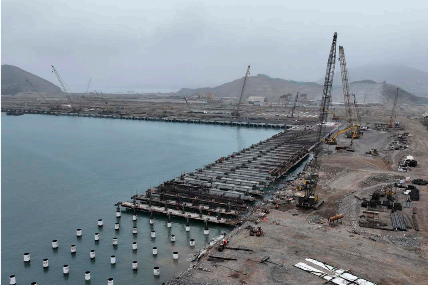
Cranes at the construction site of the Chancay Multipurpose Port Terminal in Chancay, Peru, on August 22, 2023. The Chinese state-owned company COSCO owns 60 percent of the project, which critics fear could serve military as well as commercial purposes. (Photo by Cesar Barreto/AP)
