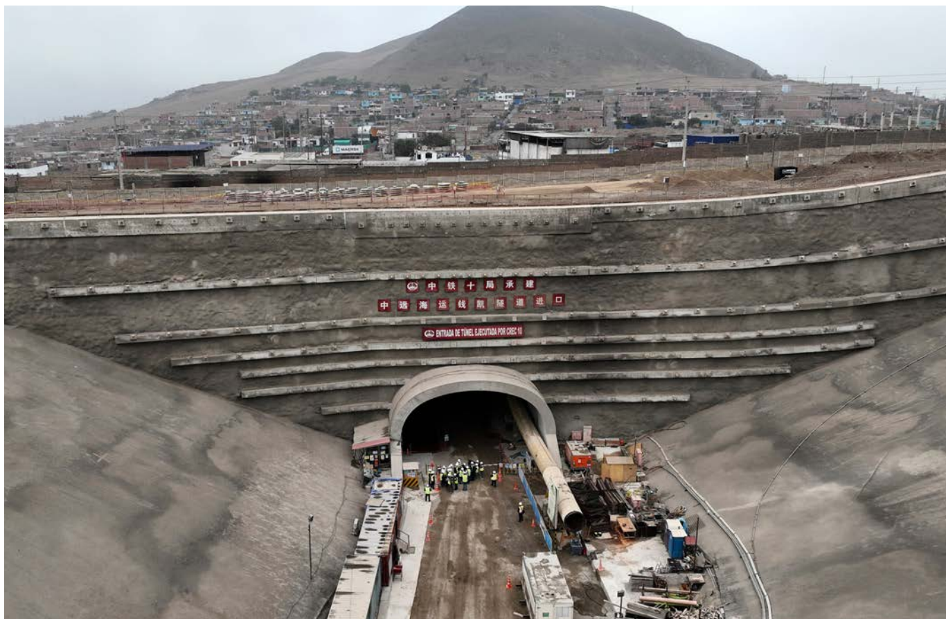
Workers building the Chancay megaport gather around the entrance of a tunnel that connects the port to the Pan-American Highway on August 22, 2023. The Chinese state-owned shipping company COSCO is a majority owner of the port. (Photo by Cesar Barreto/AP)
